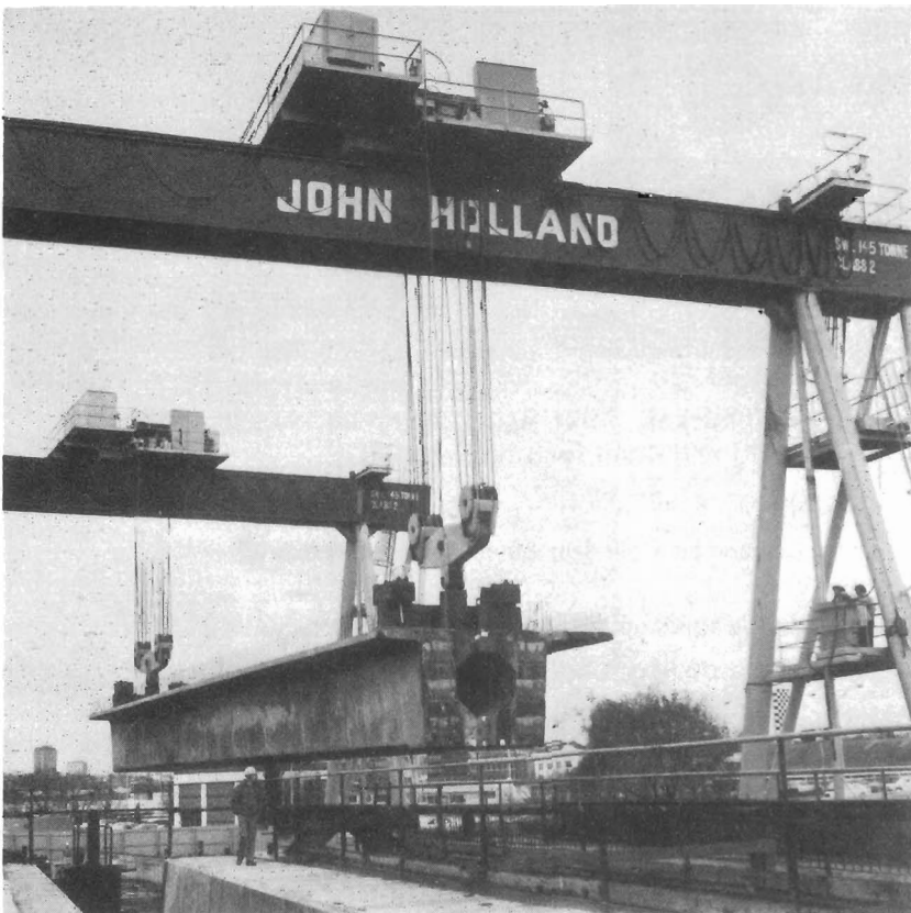
Gantry cranes lift one of the pre-cast concrete beams into position on the overpass.
