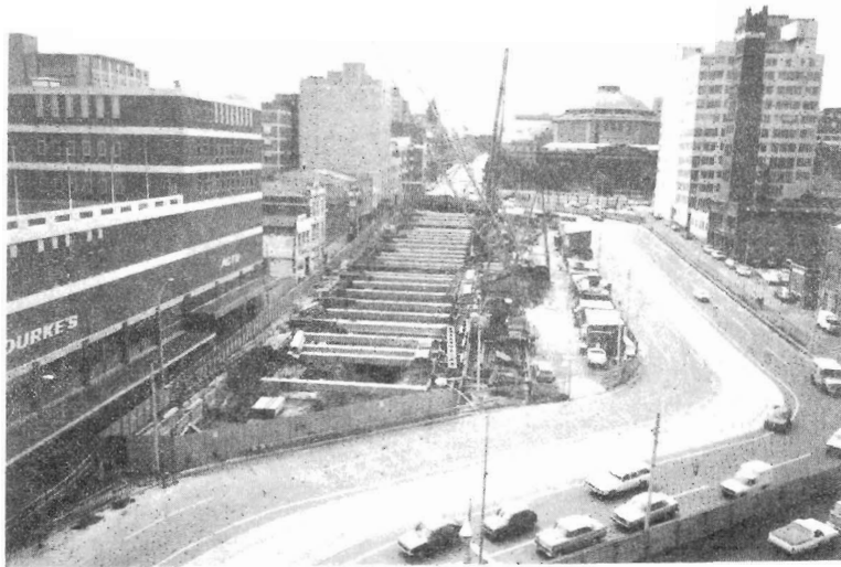
A view of the Museum station site, showing temporary road diversion and station construction work.
