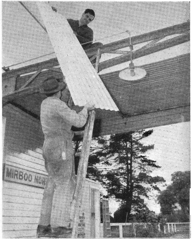
MAINTENANCE of the millions of pounds worth of Departmental buildings is a never-ending job. At Mirboo North, Plumber F. Clowes (on roof) and his assistant, L. Cottier, are renewing the roofing iron on the station verandah.
