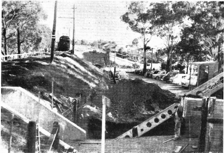
Extension of pedestrian subway and duplication of bridge at Huntingdale Road, Jordanville.
