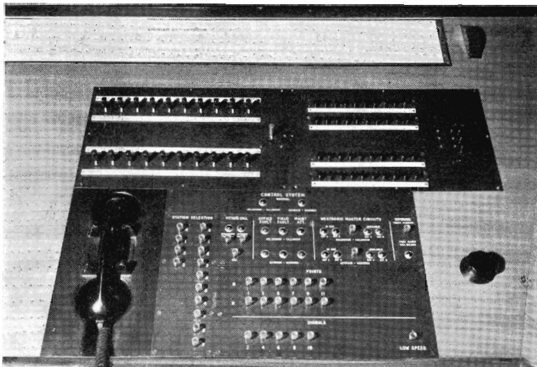
A close-up view of the console showing points and signals control panel in foreground; handset 'phone for making 'fitter's call' at left; and, in the background, a gradient plan of the line.
