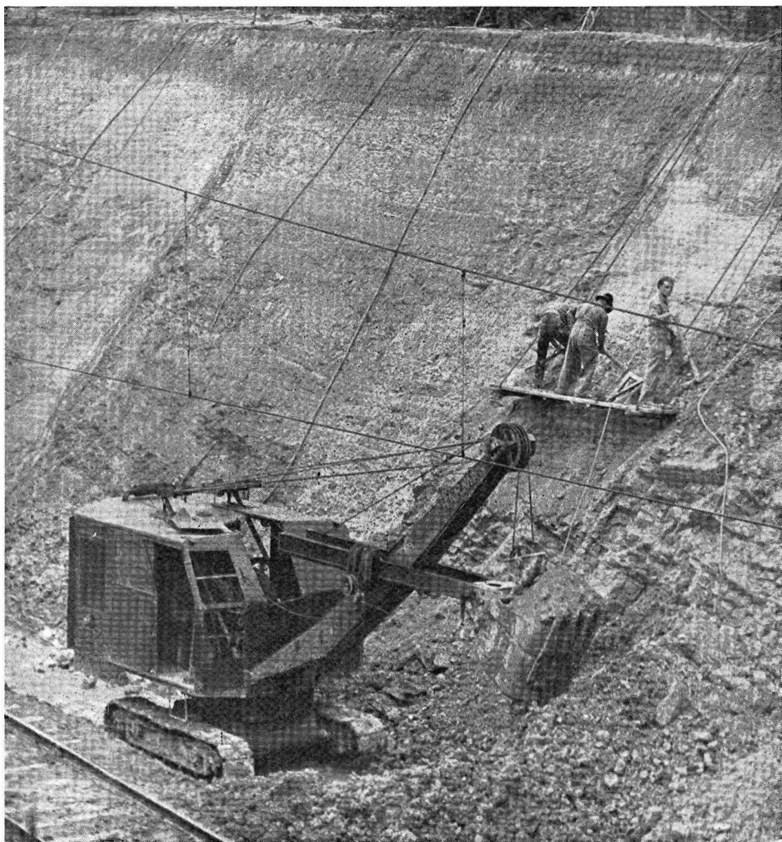
The duplication of the section of the line—a distance of 2½ miles—will greatly relieve the pressure on the Melbourne—Heidelberg line, especially in peak hours. Above is shown an excavator at work in a cutting near Darebin.
