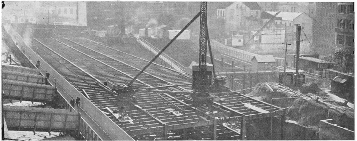
Where the roof of Wynyard station will be. The steel framing of the station is seen in the centre, with temporary footpaths laid down for pedestrians
