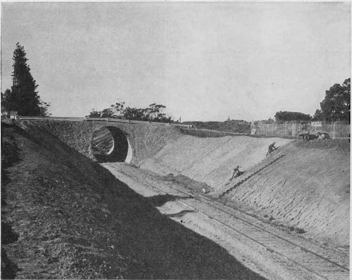
The new line to Long Island Point showing Australia's first Multi-Plate pipe structure for grade separation.
